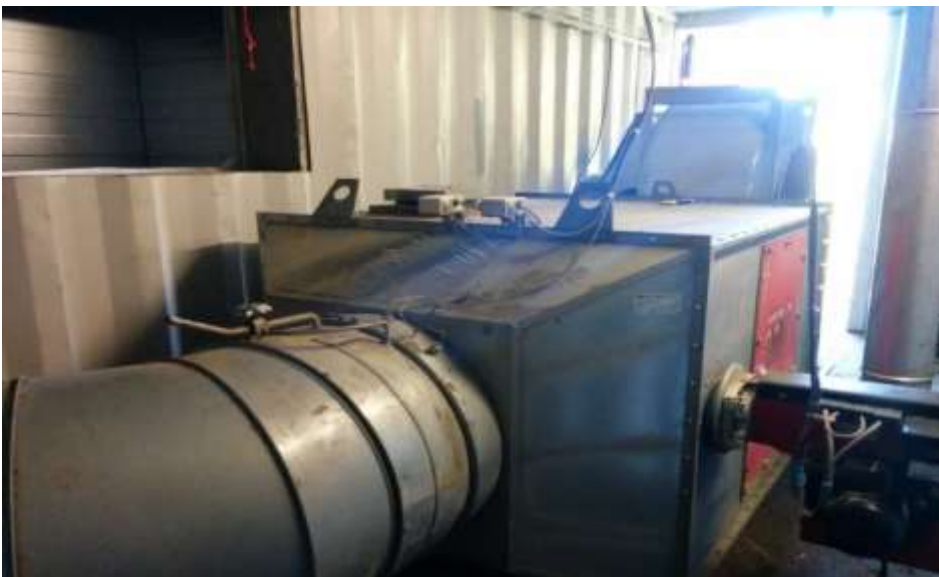
Figure 3. Blower and burner for the dryer. The opening in the upper left corner is for air intake where the residual heat from the dryer is used to preheat the air before drying.
