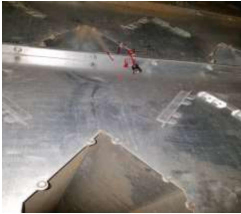
Figure 27. Location of a temperature sensor inside the dryer close to the top.
