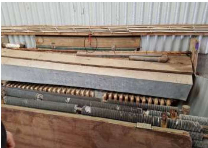
Figure 29. A heat exchanger for the dryer. A temperature sensor is located above the heat exchanger.
