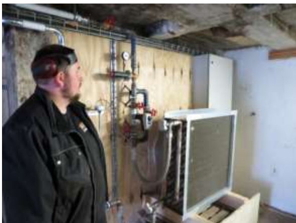
Figure 18. A heat exchanger for the incoming geothermal water.
