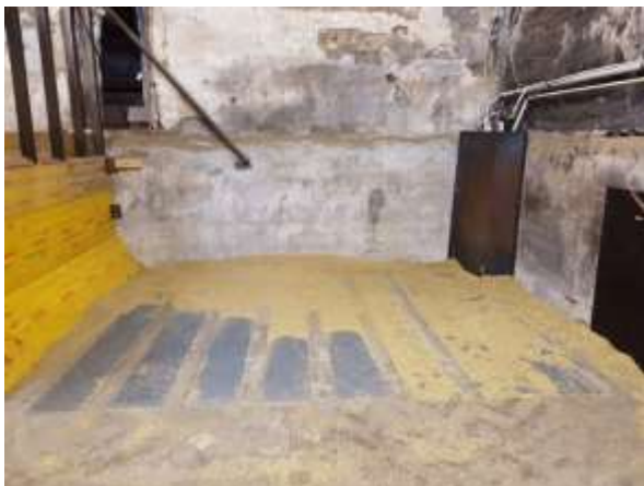
Figure 17. Facilities for incoming wet grain.
